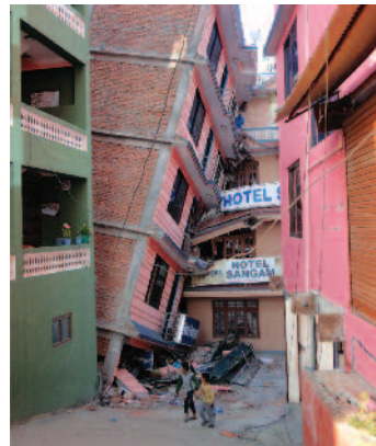
Damage to buildings in Charikot, the capital of Dolakha district in Nepal. Dolakha was badly hit by the 7.3 magnitude earthquake which hit Nepal on May 12th, causing almost total destruction of houses in some areas. Photo by Kieran McConville, June 2015.
